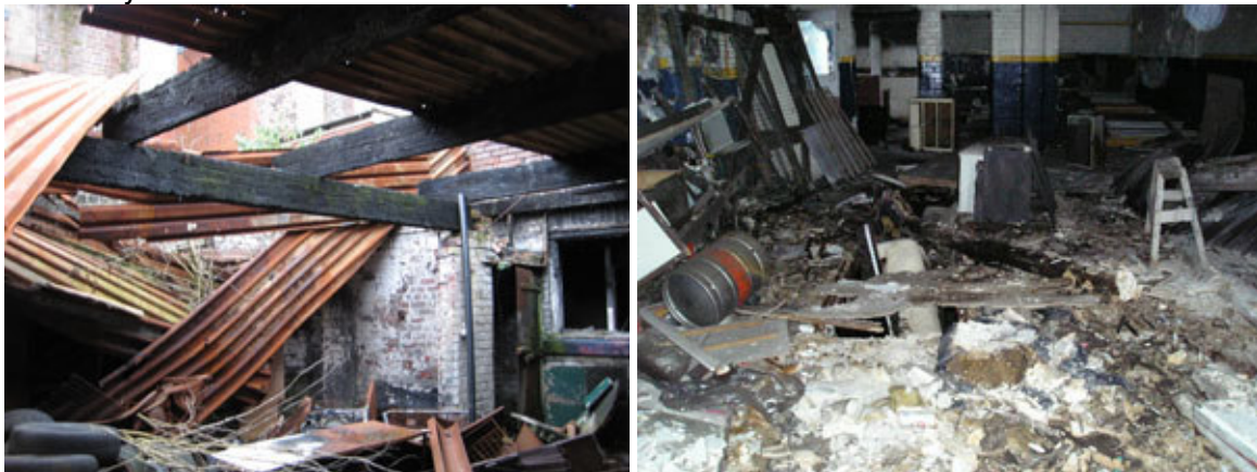
Fire damage and internal debris
